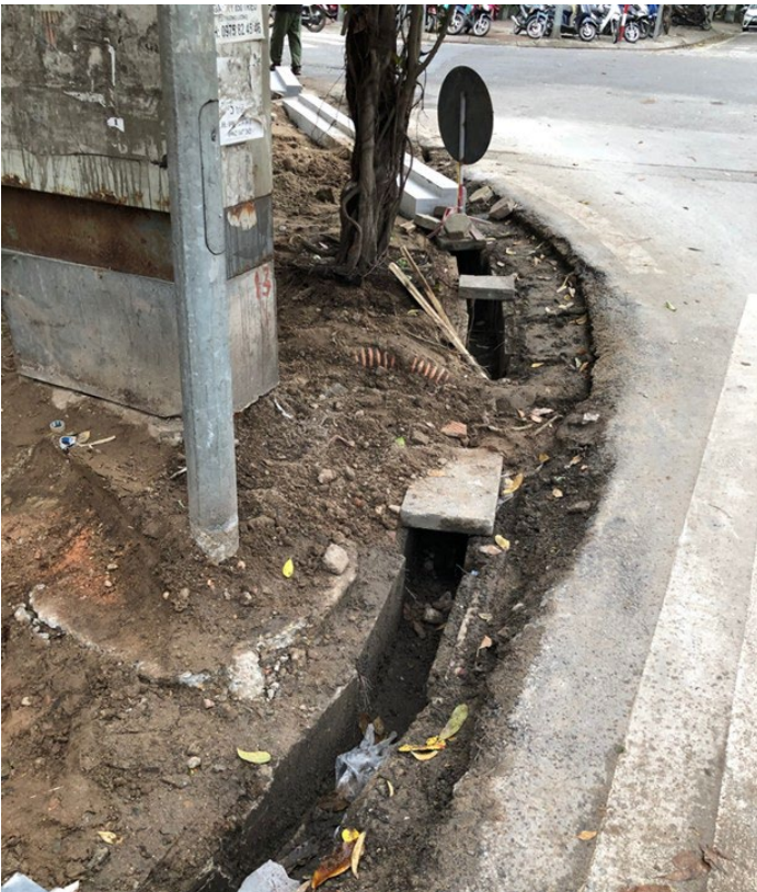
Street drain is used as a part of combined sewer network (Hanoi city, November 2020)
