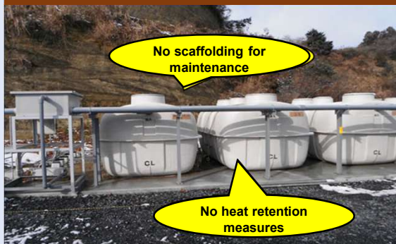
No scaffolding for maintenance No heat retention measures
