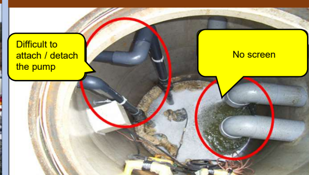
Inadequate screen equipment
