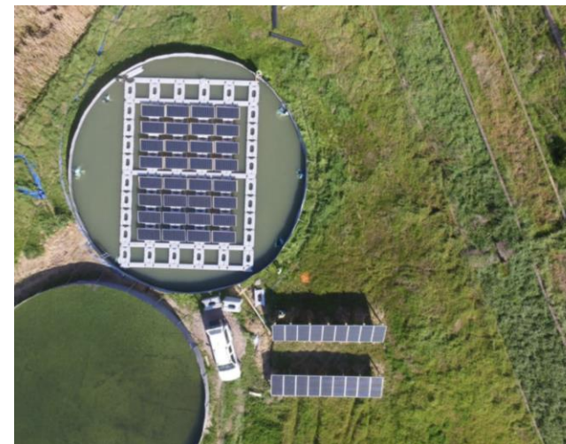
Floating Solar panels in WWTP Kraaifontein, South Africa
