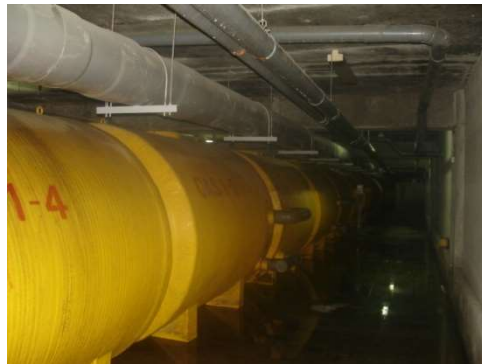
Pacific building, Hanoi 35 FRP tanks
